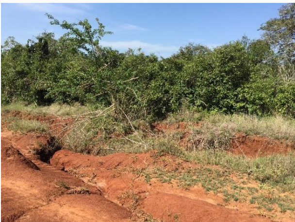
erosion resulting to deep gulleys.
